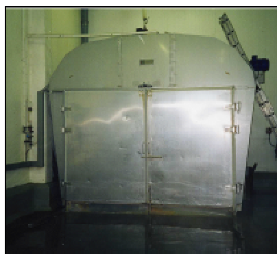
A forced air thawing unit in operation
